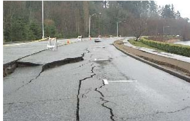
Figure 4.G2-3 Lateral Spreading –March 2001
