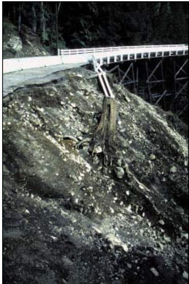
Figure 4.G3-3 SR-165 Bridge along Carbon River – Landslide 2/1996
