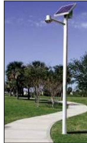
Solar pedestrian scale light Source: Sol Systems
