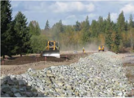
Pierce County built the Soldiers' Home set-back levee in Orting in 2006 to help reduce flood damage from the river.
