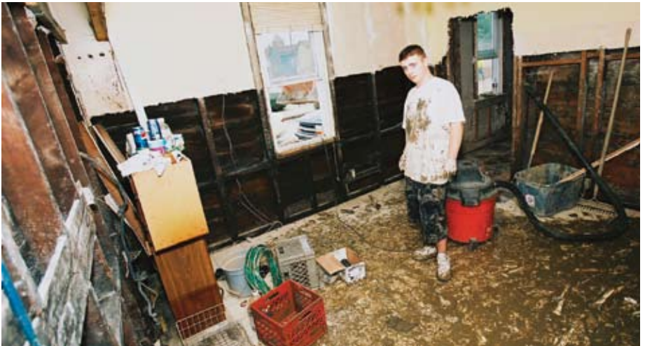
Thoroughly dry out your home to reduce mildew damage.
