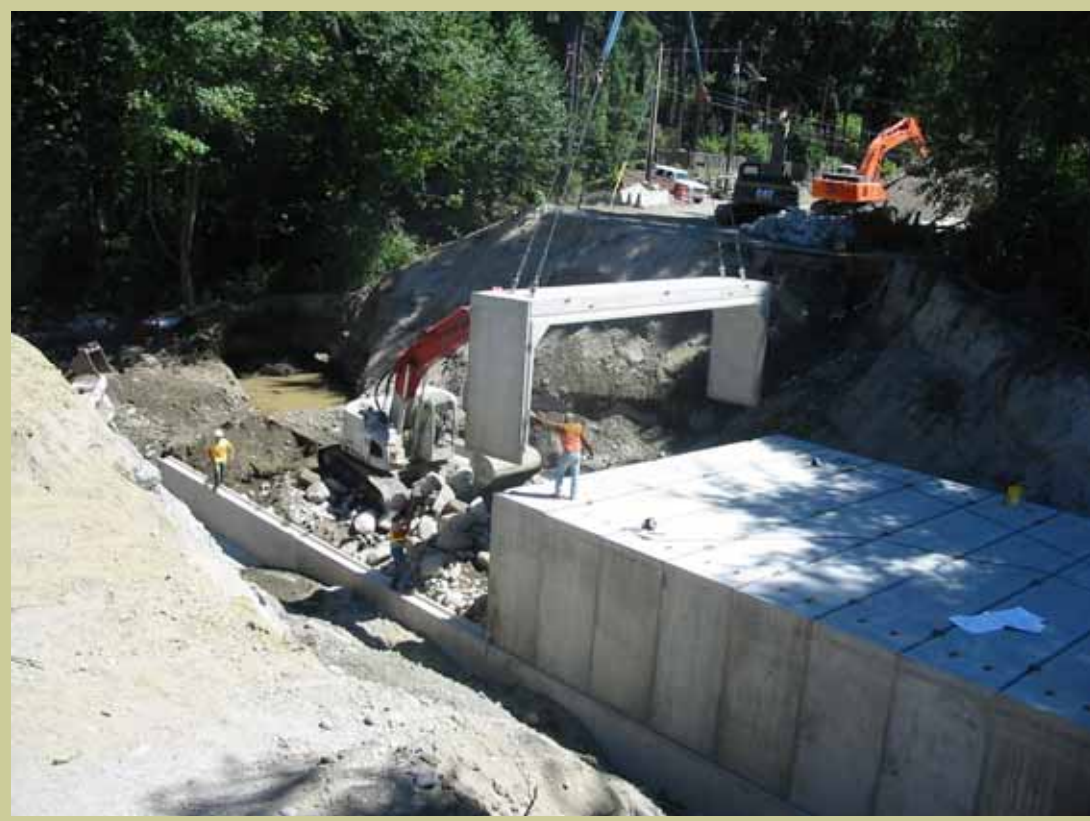
SRFB-funded box culvert installation to improve fish passage in Leach Creek, under Bridgeport Way SW, University Place. July 2005.
