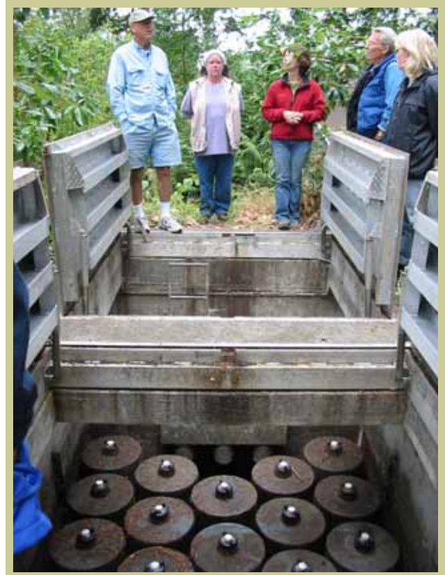
Stormwater filtration vault near Lake Louise, Lakewood. Sept 2006.
